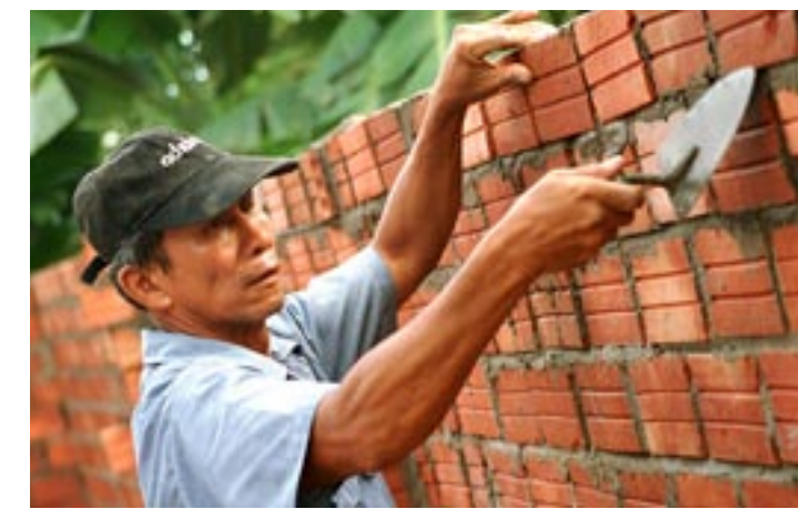
A man works on the wall of a house in Vietnam. Since 2002, Vietnam has been the site of a successful Save & Build program.
